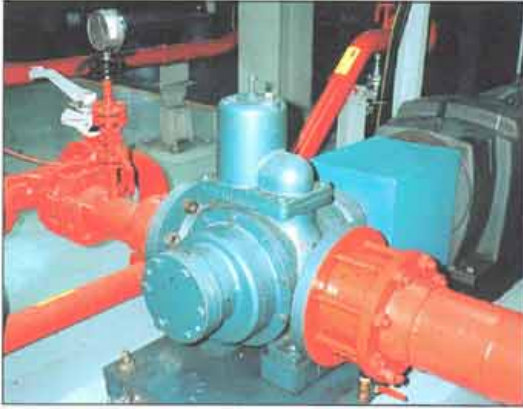
G2000 Lubricants Transfer Pump connected to piping with compressed air purge and pigging system.
