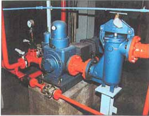
U2000 Pump with Gas Loaded Constant Pressure Control pumping Lube Oil to drum filling machine.
